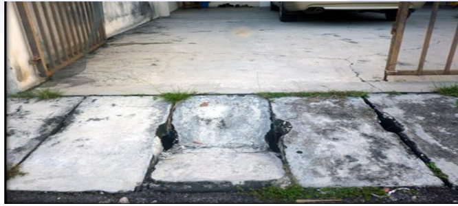
Figure 4. Damage to concrete cover
