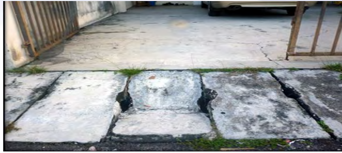
Figure 4. Damage to concrete cover
